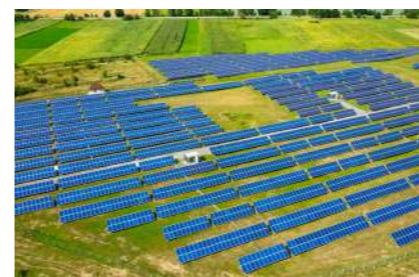
Solar Farm Project (Bambous, Mauritius)
